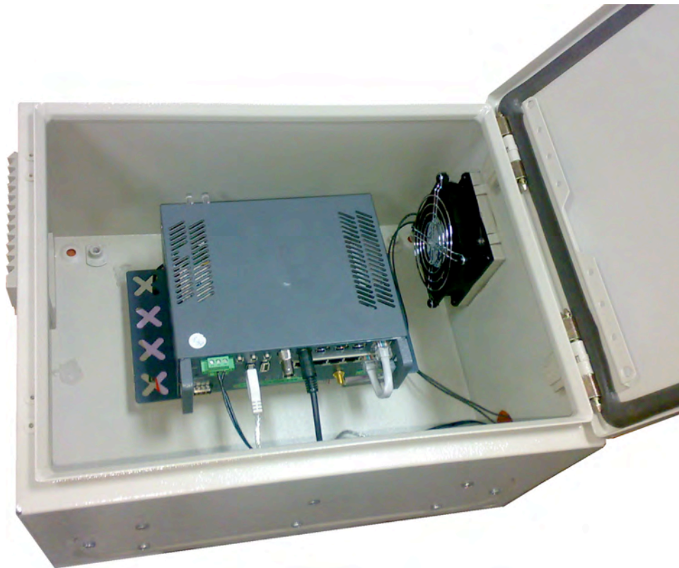
Figure 1: TVG unit installed in an insulated container
