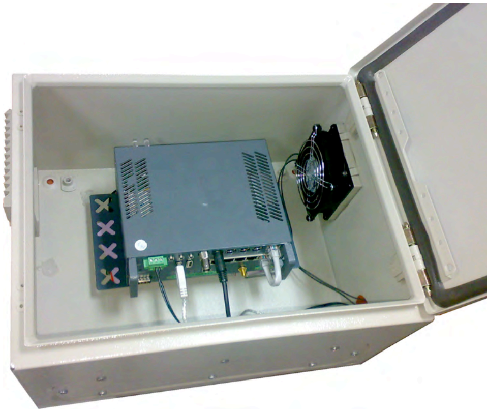
Figure 1: MVG installed in an insulated container
