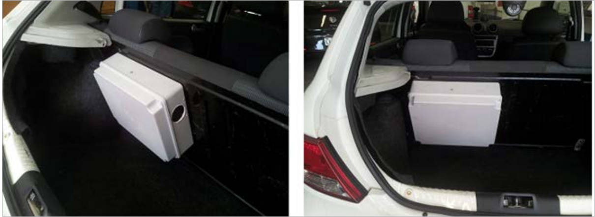
Figure 2: Video Gateway installed in an insulated container attached to the back of a seat in a car
