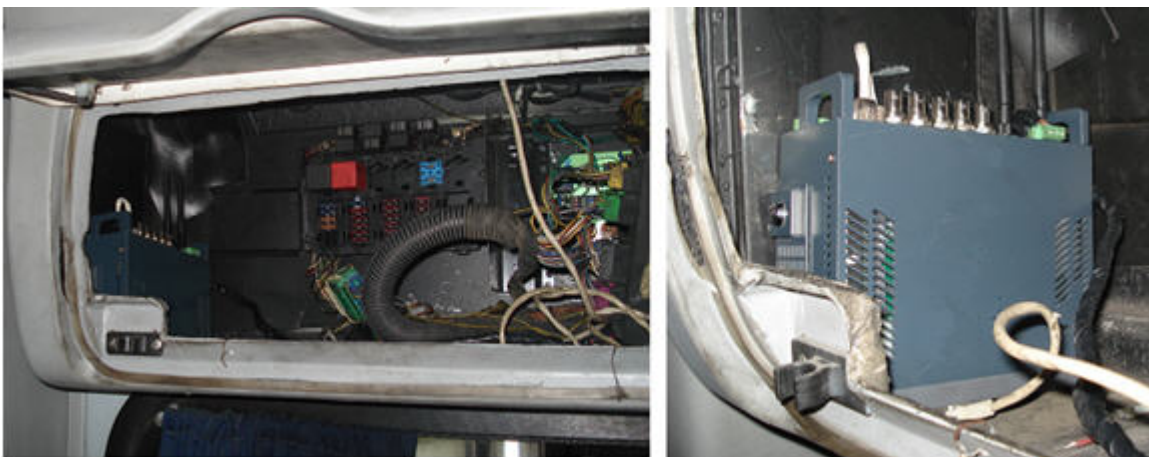
Figure 4: Video Gateway installed in the compartment above the driver's seat in a bus
